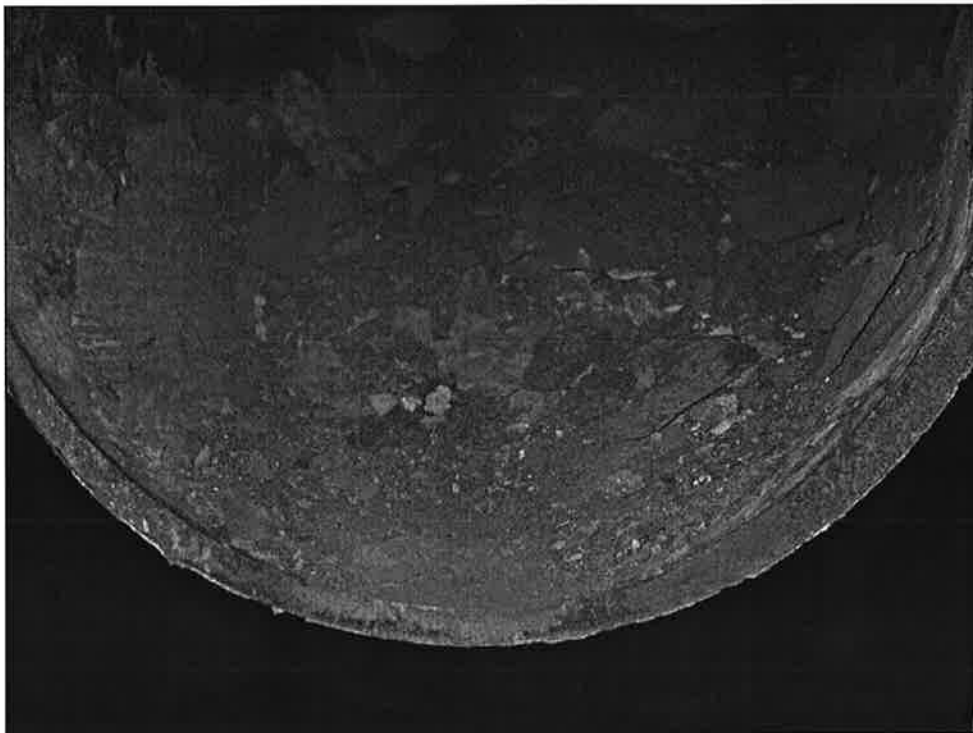
Fig. 9: Photo showing the scale flakes of corroded material at A-5. Note the black colour of the flakes.
